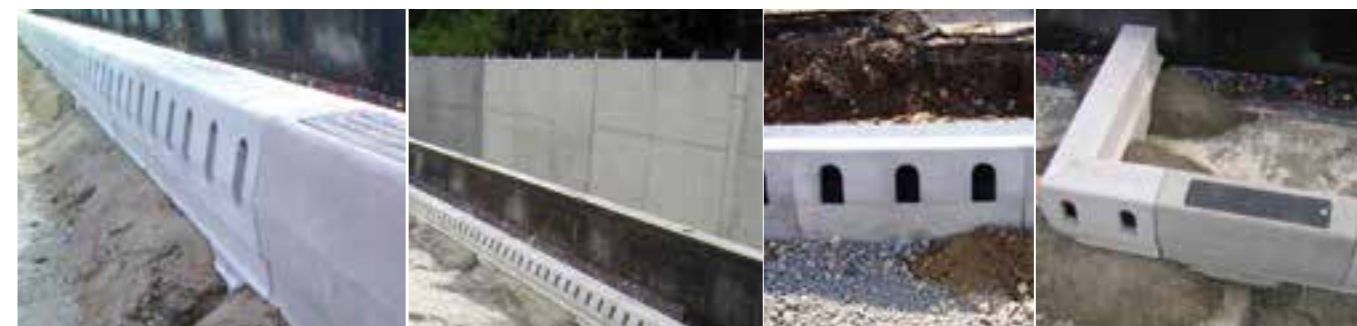
If there is a layer of asphalt behind the units, the concrete can be adapted by lowering the concrete side. All the stone pavement blocks adjacent to the kerb must be secured with modified polymer or epoxy mortar.
