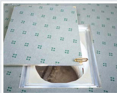
BVA installed in an office (over a manhole), in a carpeted area
